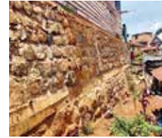
The construction of this supporting wall was necessary to support the original foundations of the school in Ciriri | K 04
